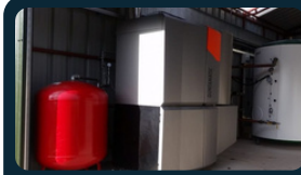
Biomass Heating and Heat Pumps
