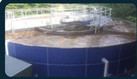
Activated Sludge Treatment
