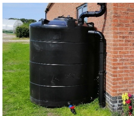
Rainwater harvesting tanks are positioned at key downpipe interception points around the farm buildings.
