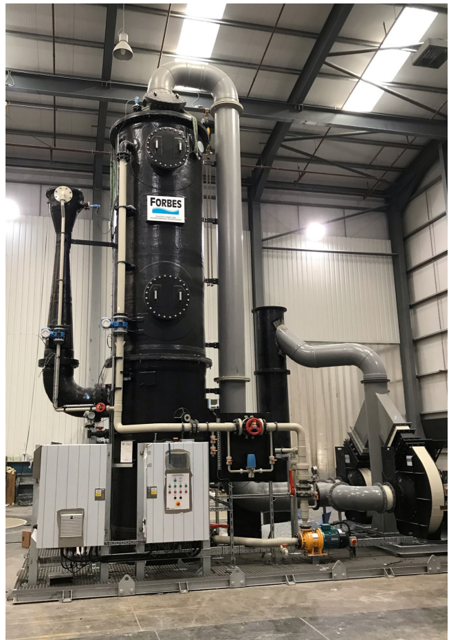
Skid-mounted scrubbing system
