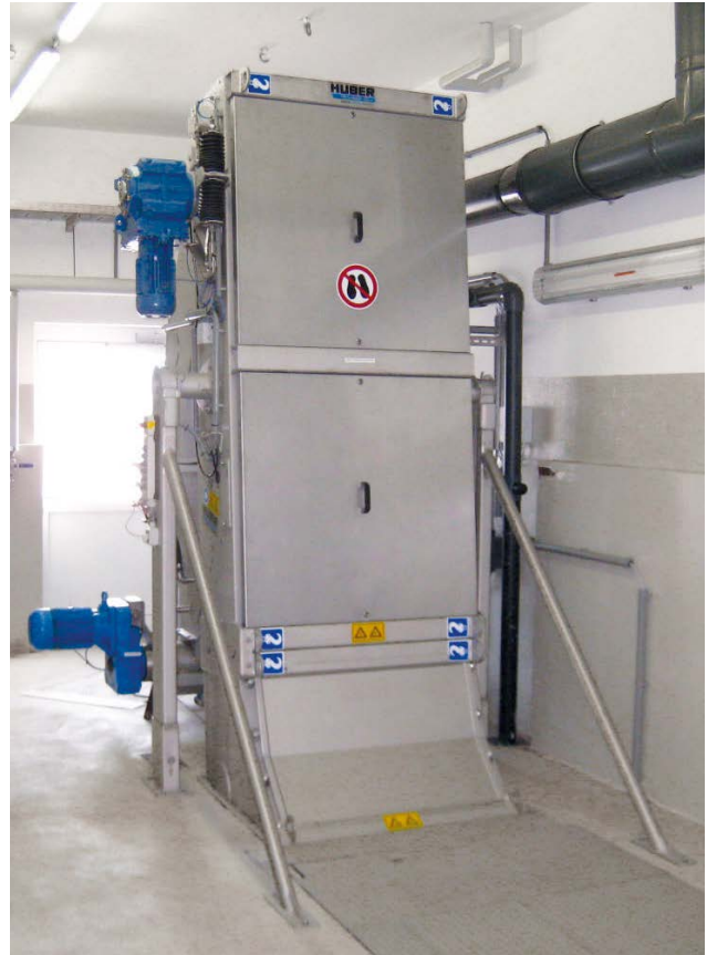
Installed HUBER Multi-Rake Bar Screen RakeMax® HF.
