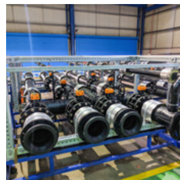
Roof top modules
