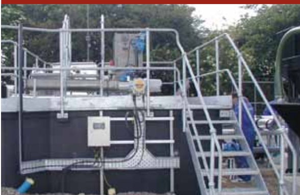
A J+A CIS for 140 l/sec, featuring a full carbon steel design and partly buried below grade
