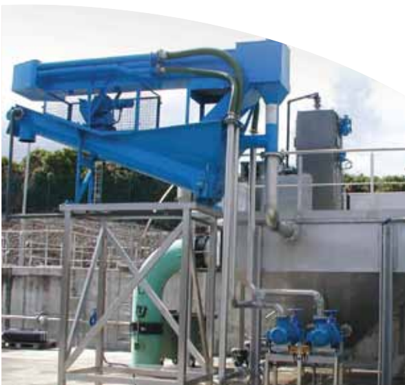
A typical J+A CIS, manufactured from stainless steel. Handles a flow of 135 l/sec
