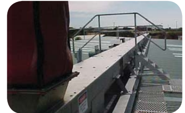
Long continuous sludge run
