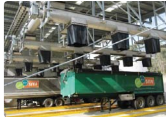
Truck outloading system
