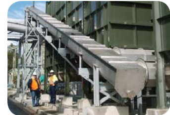
High capacity sludge outloading system
