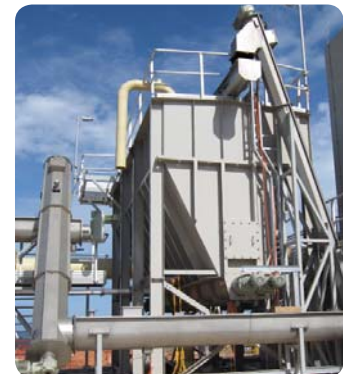
72 degree and 40 degree inclined OK trough sludge conveyors
