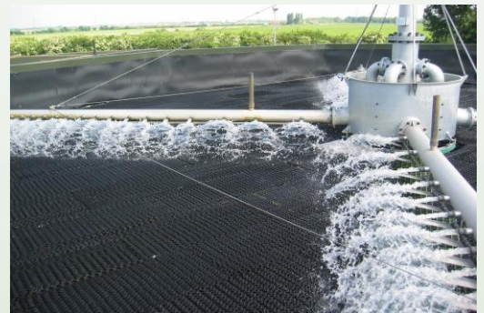
4 Arm motor driven HYCOVER tubular arm distributor applying some 170 lt/sec to 12.0 mt dia HYRATE nitrifying filter.
