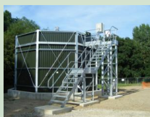
Typical HYRATE Polytower with stairway and local control panel on top platform adjacent to doorway
