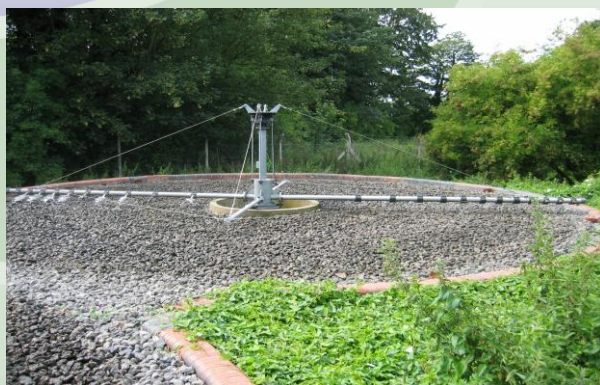
2 Arm reaction driven HYCOVER 'Lo-Flo' tubular arm distributor applying 3.2 lt/sec to an 18.0 mt dia stone trickling filter.
