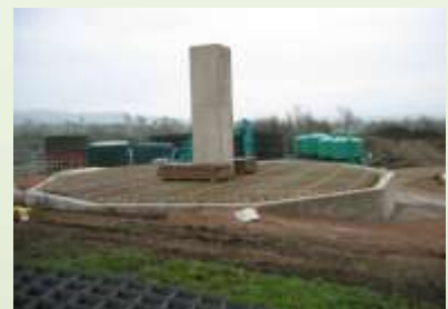
Timber matrix modules in place ready for construction of new HYRATE Polytower filter shell.
