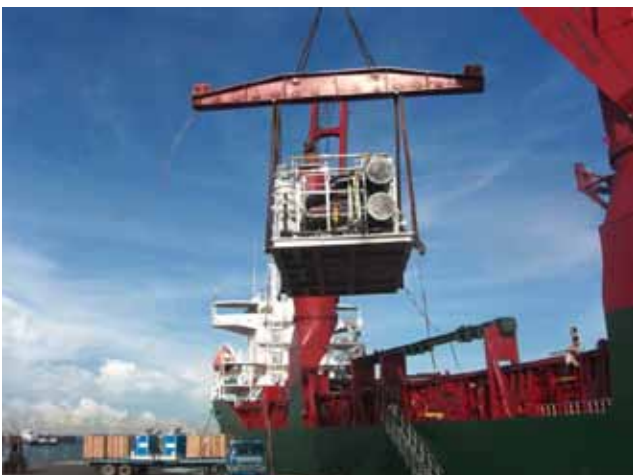
Below: TOTAL Usan Offshore Oil Field Project West Africa NIGERIA Protection of S.R.P. Sulphur Reduction Package
