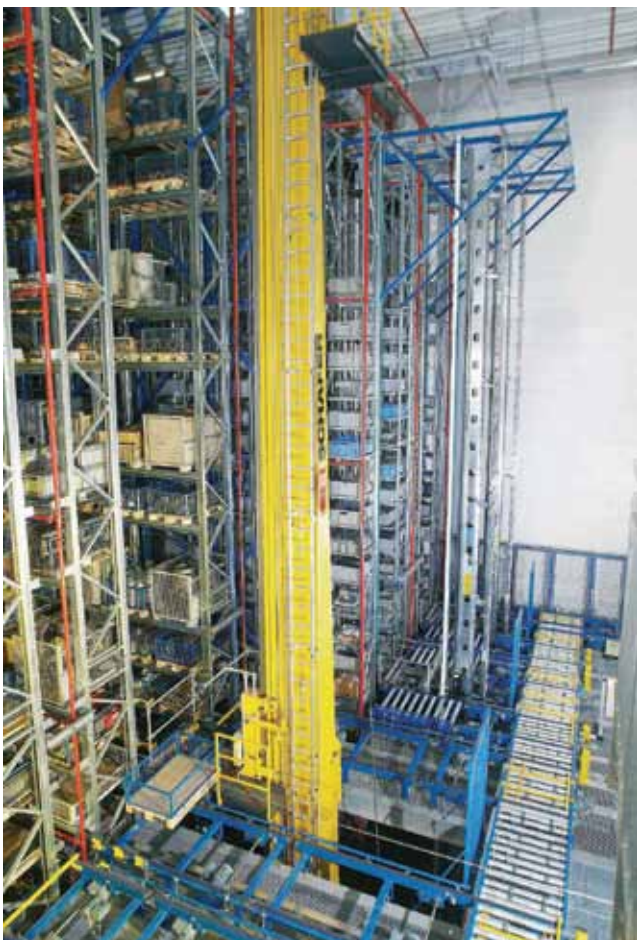
Automated racking in computer-controlled storage area
