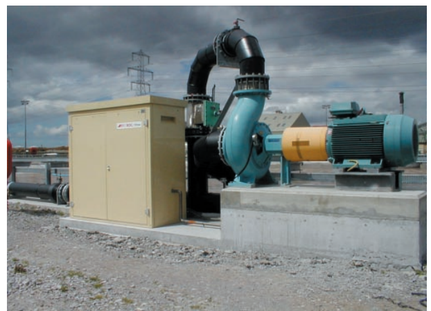
Vitox pump alongside oxygen control kiosk at Shotton Paper
