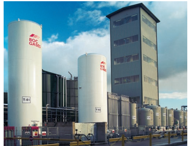
Oxygen vessels, ammonia stripping columns and Loprox unit
