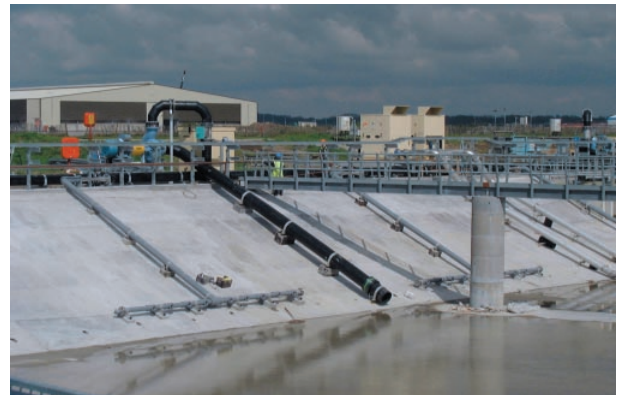
Sparger pipework in the lagoon at Shotton Paper
