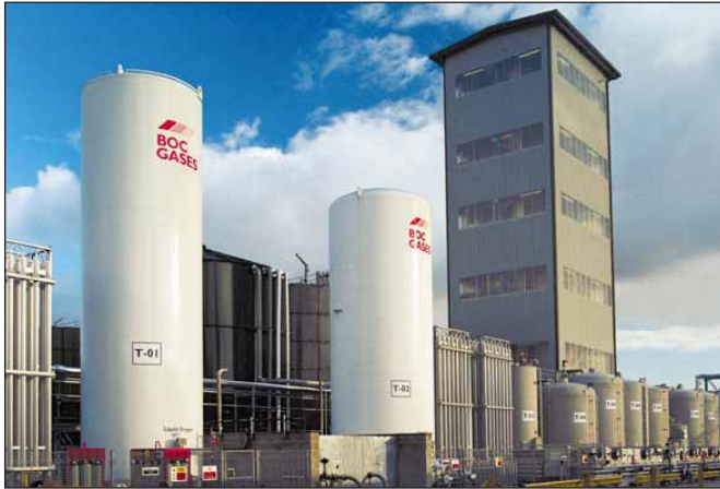
Oxygen Vessels, ammonia stripping columns and Loprox unit
