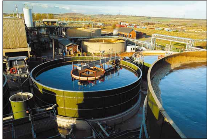
Vitox biological plant
