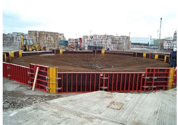
22 m diameter Clarifier
