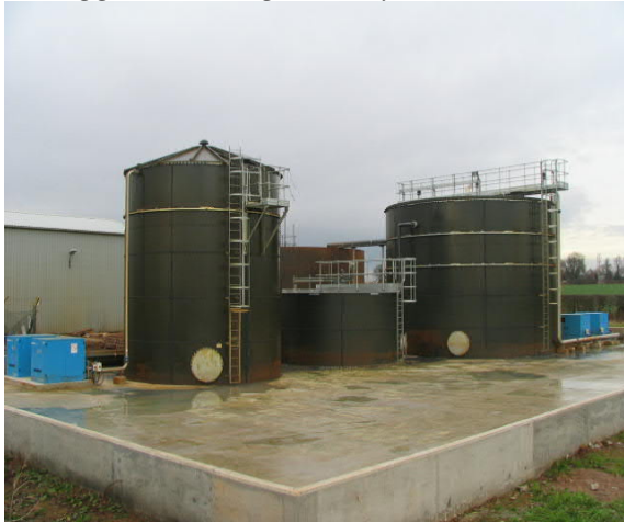
500m 3 /day Full Treatment to Sewer
