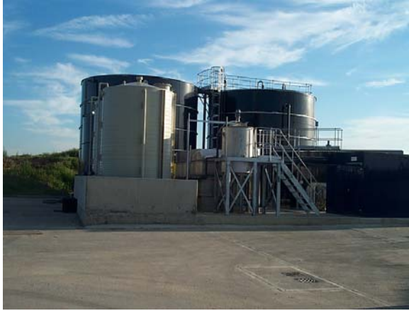
720m 3 /day Biological Treatment Discharge to sewer
