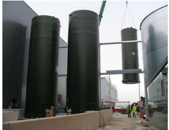
100 m 3 /hour effluent balancing And pH correction
