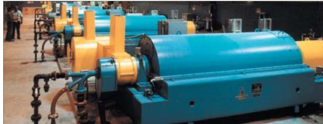
Multiple centrifuge installation
