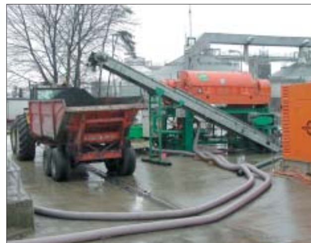
Packaged centrifuge plant
