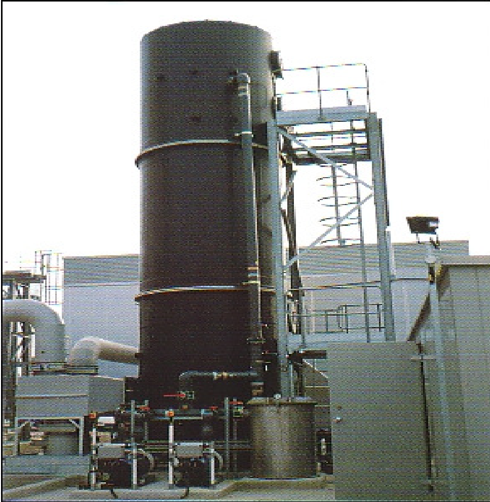
29,000M 3 /HR Odorgard unit supplied to Southern Water
