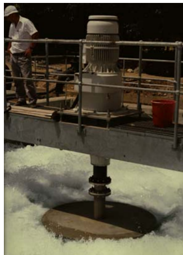
Surface Aerator - Municipal
