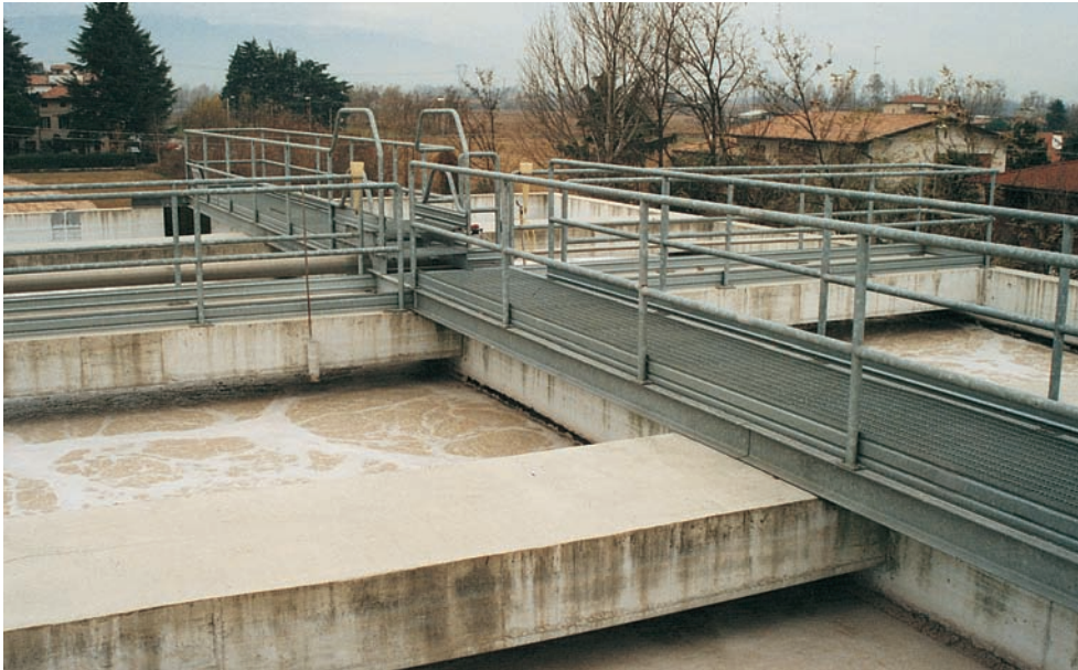
Activated sludge plant
