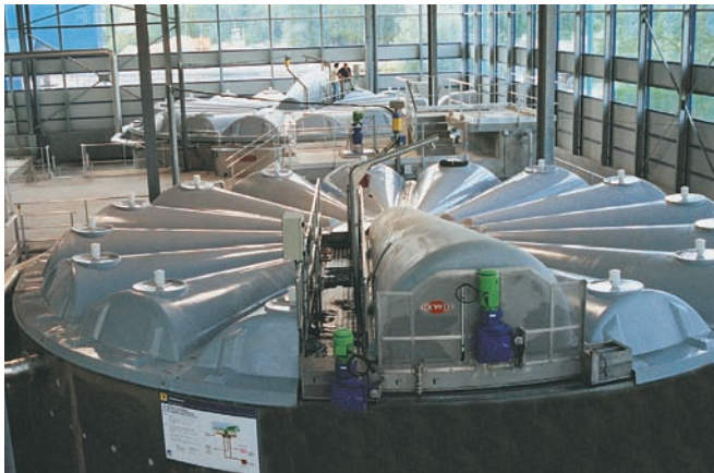
Biobuffer backwash water clarification and sludge thickening
