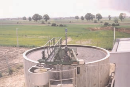
Biological sludge thickening, dairy
