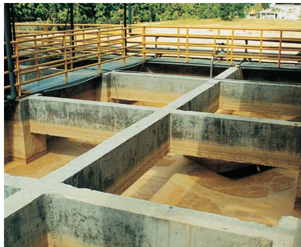
Sequential batch reactor (SBR) - rubber manufacture
