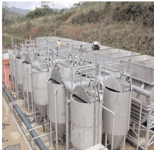
Turnkey drinking water project - with lamella settlement and sandfiltration
