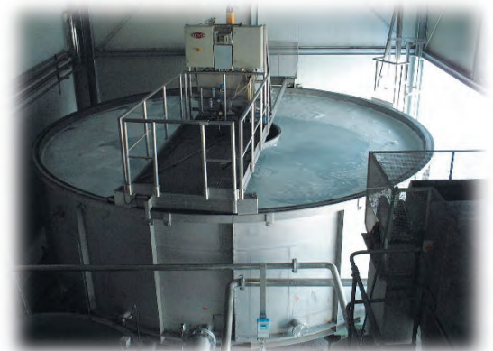
KLC 24 - Process water treatment textile industry
