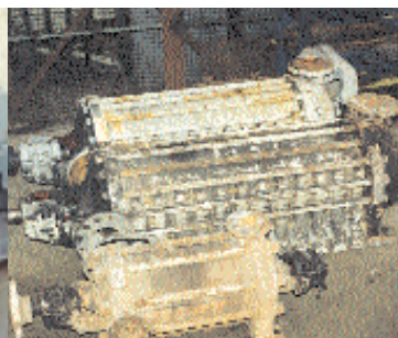
Multi-stage dewatering pump before overhaul...
