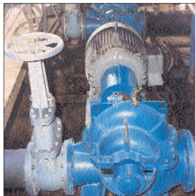
A split case cooling circulation pump
