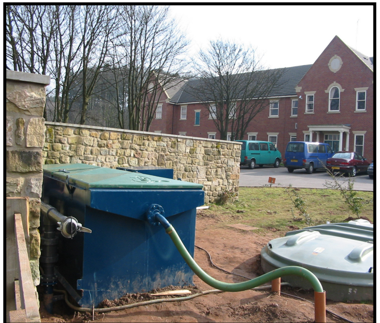
Pollution Control's Nitrification unit (shown on left) greatly enhances the nitrification process which the original RBC (shown on right) was failing on. The plant is now screened from view by conifers and bushes.
