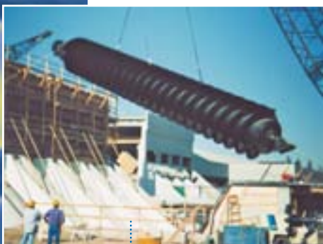
Archimedian screw pumps
