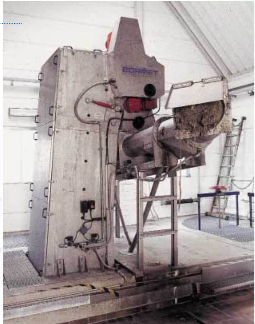
Washing compactor with fine screen
