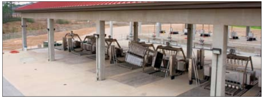
The eight TrojanUV4000Plus™ reactors used to disinfect 600 MGD (94,680 m 3 /hr) at this large wastewater treatment facility require a footprint measuring only 80' x 120' (24 x 36 m) – a fraction of the space needed for chlorine disinfection.
