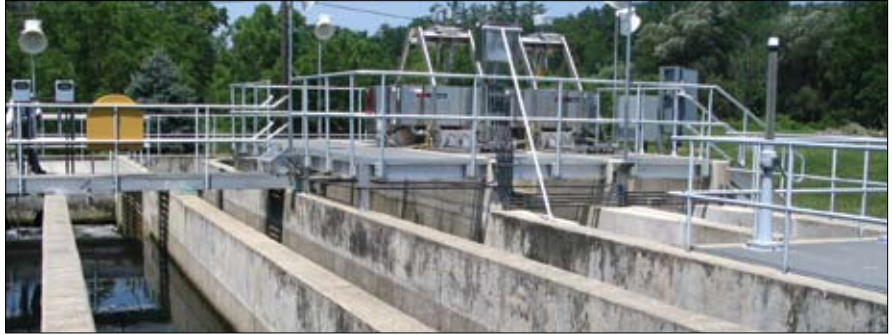
In this retrofit installation, each reactor was installed in one pass of the existing chlorine contact basin with only minor modifications to the channels. This allows the majority of the basin to be used for storage, by-pass or emergency back-up.
